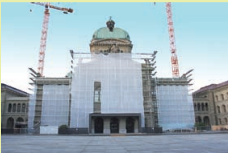
Under construction – Swiss parliament has not come to term with its climate policy yet.
