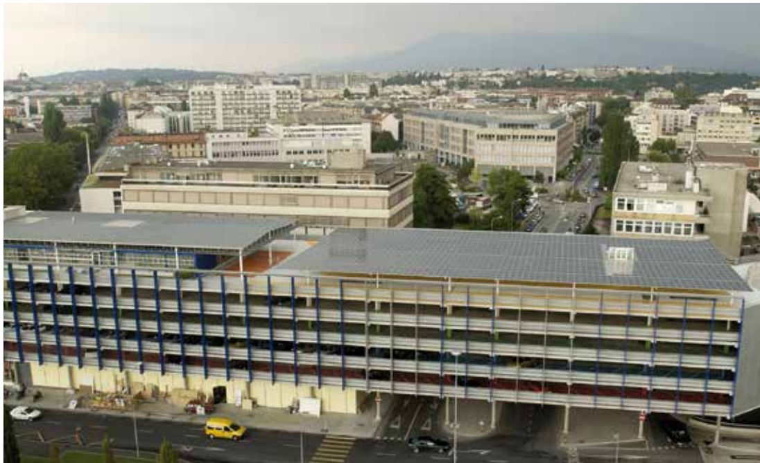
Figure 3: Photovoltaic system installed on the «P+R de l'Étoile» car park in Geneva. Foto: Services industriels de Genève, SIG.
